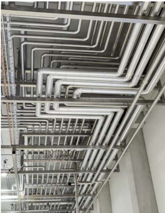
The part of Möstl Anlagenbau consisted of the entire energy supply as well as the installation of the tank farm and the CIP system including the piping (photo: Möstl)
